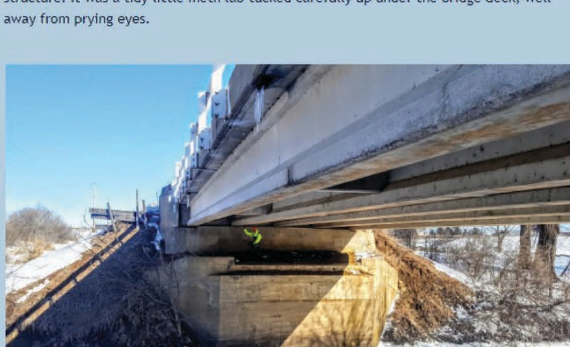
WHKS inspectors work to get views of all areas of the bridge, even when special access equipment isn't available.
