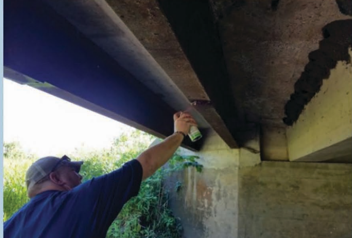
An inspector performs dye-penetrant testing to check for cracks that aren't visible to the naked eye.
