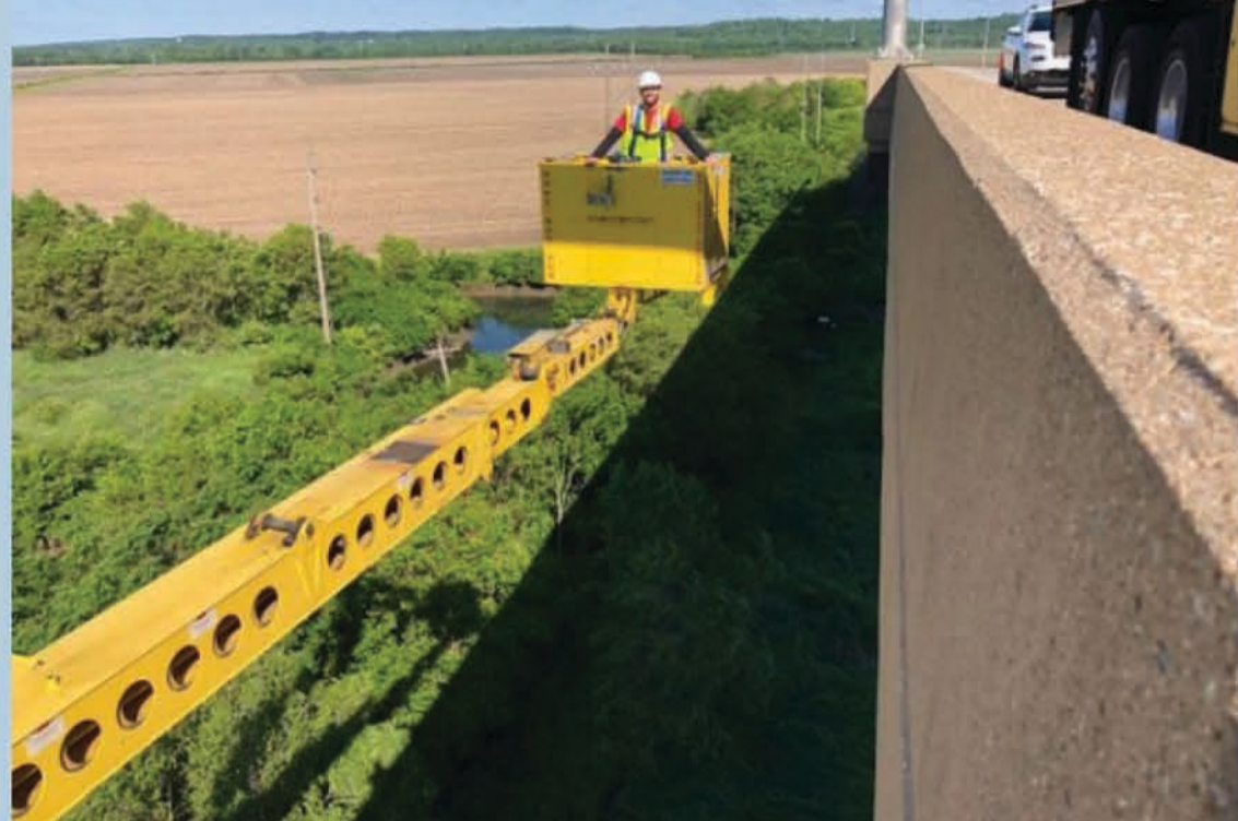
Bridge inspections can involve a variety of equipment as well as a wide range of structure types.
