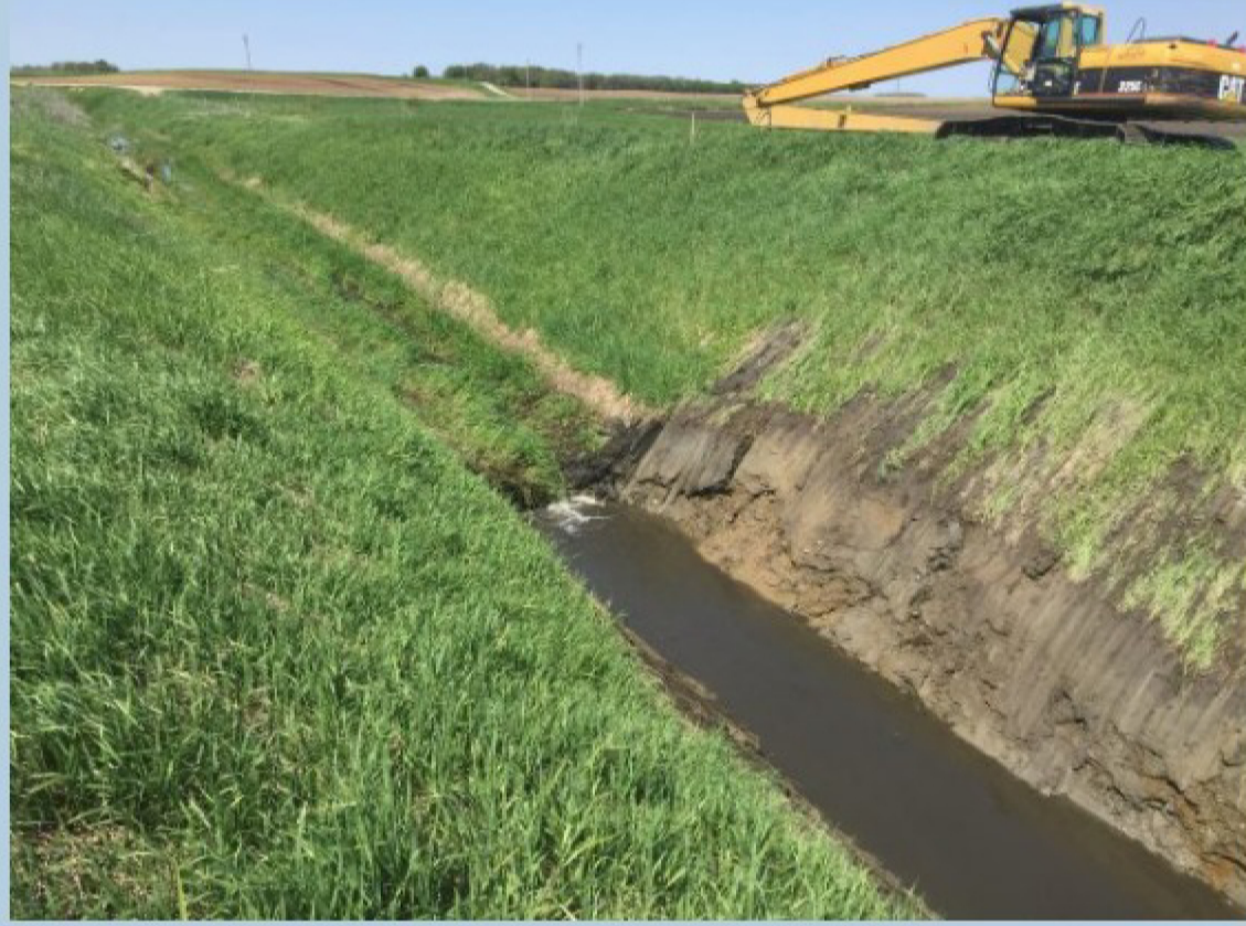
An example of the amount of siltation that occurs in drainage ditches over many decades.
