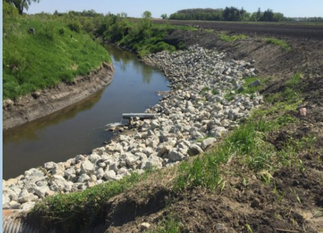
Drainage Ditch cleanout, repair, and protection at an outside curve of a drainage ditch bank.
