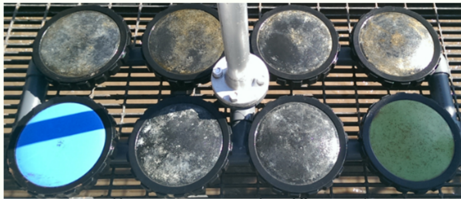
Field test unit in service to evaluate different membranes
