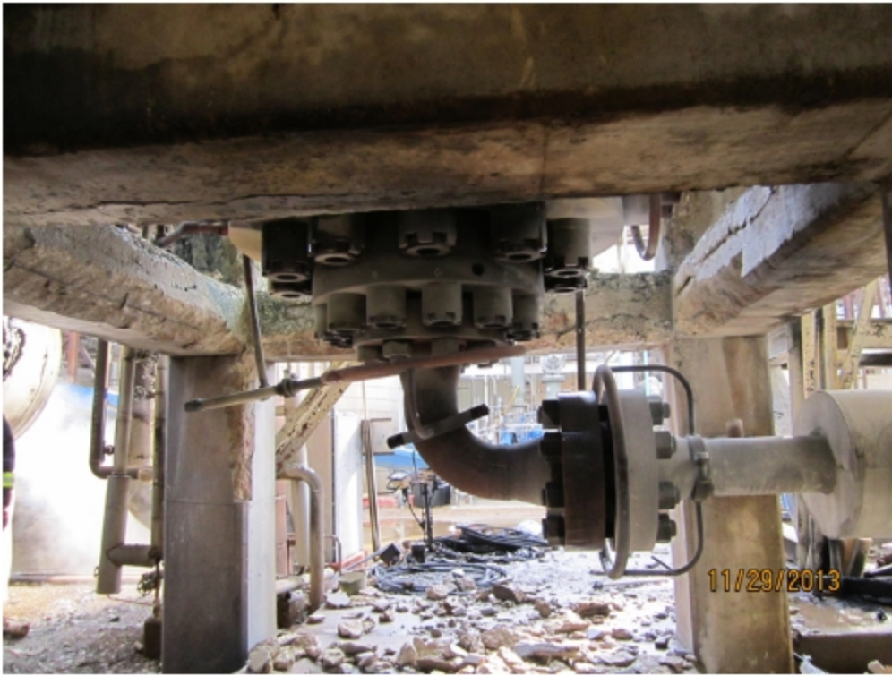
Fire Damaged Concrete Structure Supporting 225-Ton Vessel
