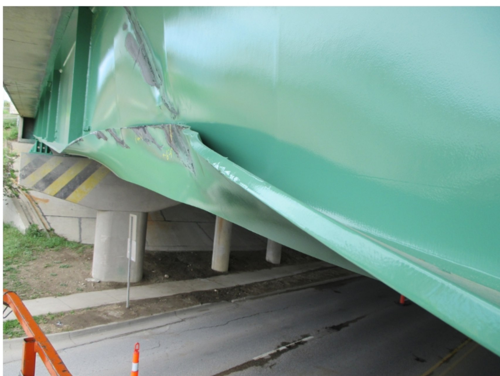
Ramp B south girder collision damage close-up
