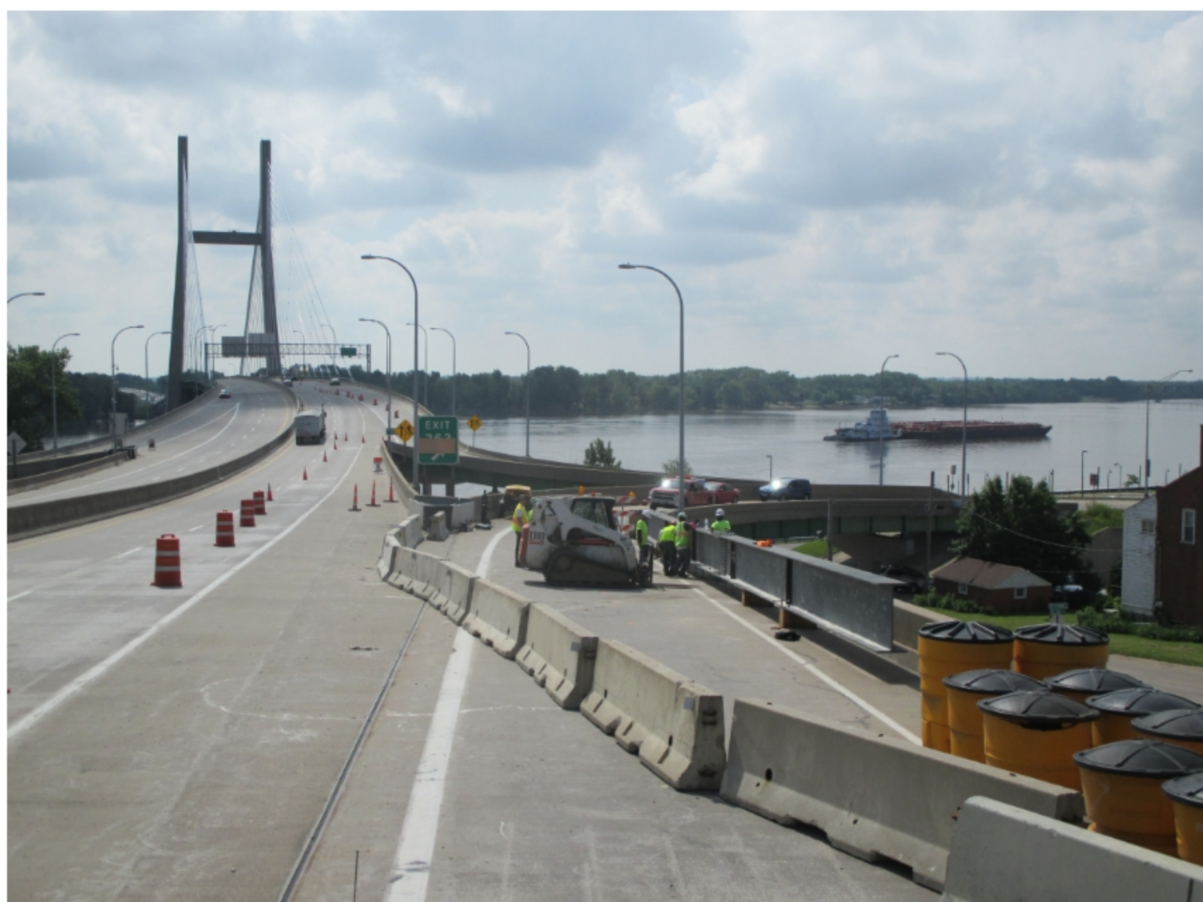
Installation of strong back beam over south girder of Ramp B, Phase 1
